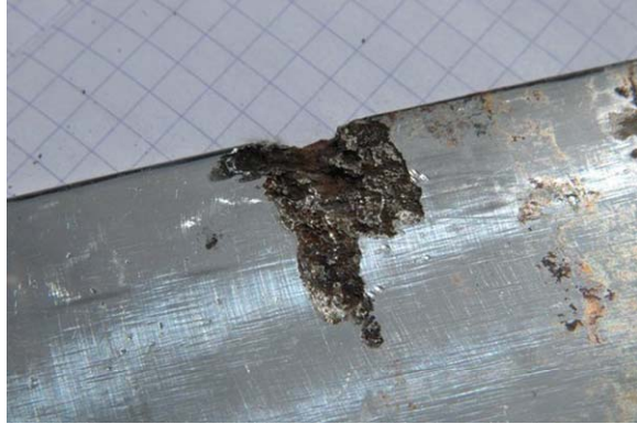
Serious Crevice Corrosion
